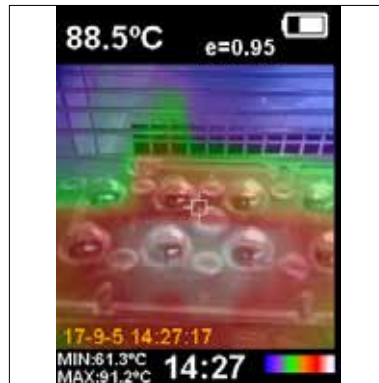
Temperature detected on the part by IR thermal camera
